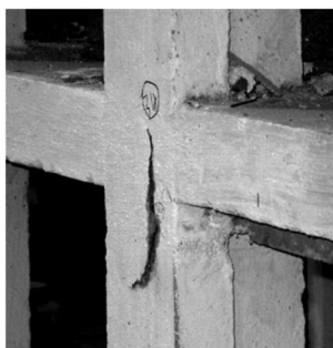
图 5 节点附近混凝土剥离 Fig 5 Concrete spall near joints
